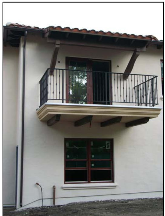
Above: Workers add finishing touches to an apartment balcony. The light, cream-colored “color coat” highlights the terracotta tile roof and charming wrought iron railings.
